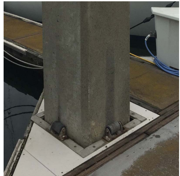
Fig. 5. Typical roller-type pile guide configuration for California small craft harbors. (Image by Adam S. Keen.)
