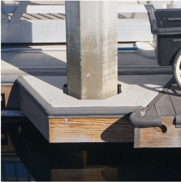
Fig. 6. Typical high-density polyethylene (HDPE) pile guide configuration for California small craft harbors. (Image by Adam S. Keen.)
