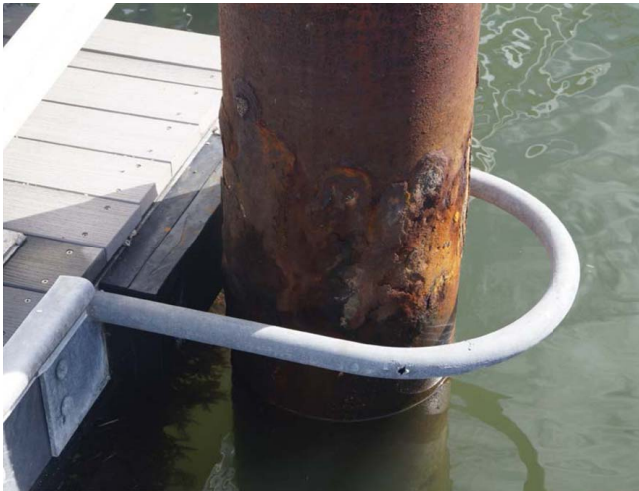
Fig. 4. Typical hoop-type pile guide configuration for California small craft harbors. (Reprinted from Keen et al. 2017, ©ASCE.)
