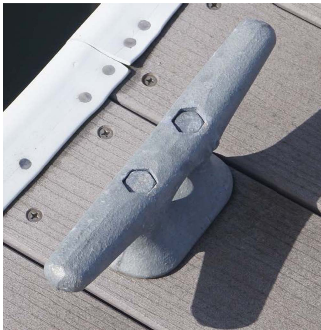
Fig. 3. Typical cleat configuration for California small craft harbors. (Reprinted from Keen et al. 2017, ©ASCE.)
