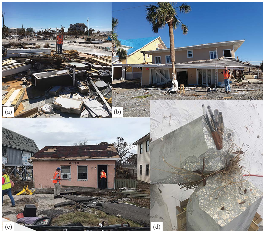
Fig. 7. (Color) Examples of structural damage: (a) destruction of at-grade house (DS6); (b) at-grade house detached from its foundations by waves and surge (DS6); (c) damaged at-grade house (note sheets of asphalt detached from road) (DS3); and (d) failure of prestressed concrete piling (DS6). (Images by authors.)
