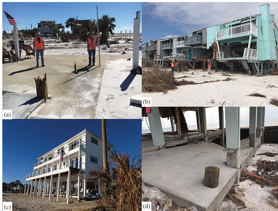
Fig. 8. (Color) Examples of structural damage: (a) complete failure of pile elevated house (DS6); (b) severe damage to beachfront pile elevated row houses (DS5); (c) minor damage to Sand Palace (DS3); and (d) scour and partial failure of concrete floor pad underneath pile elevated house (DS5). (Images by authors.)
